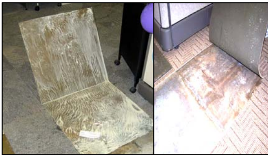
Substrate Moisture Issues
